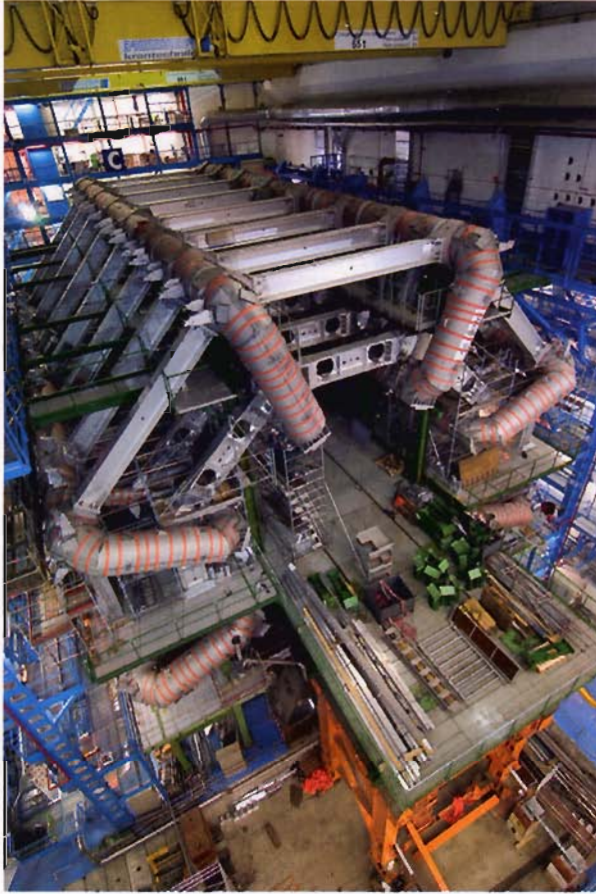
View of the ATLAS cavern with its eight barrel toroids installed and fixed
